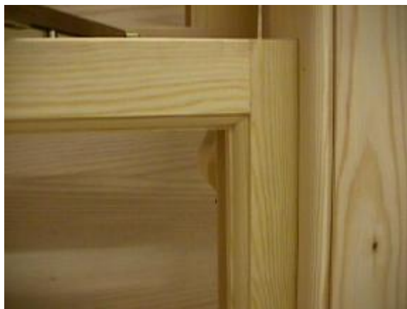
Mortice and tenon construction with ovolo scribed joints, traditional staff bead mould internally
